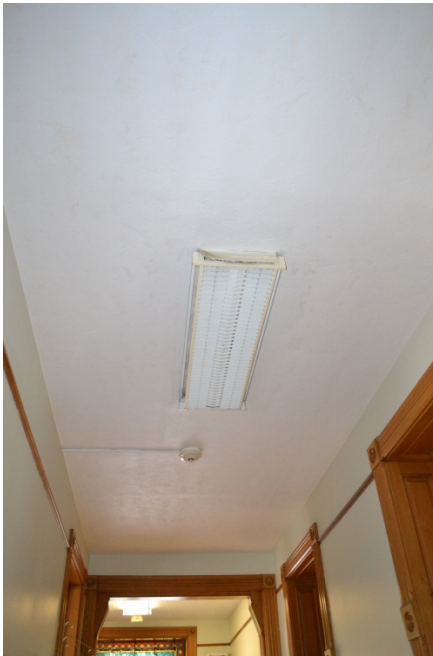
Plaster ceiling at first floor hallway
