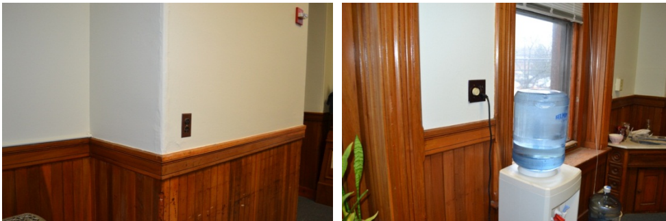
Electrical at masonry wall in the second floor conference room
