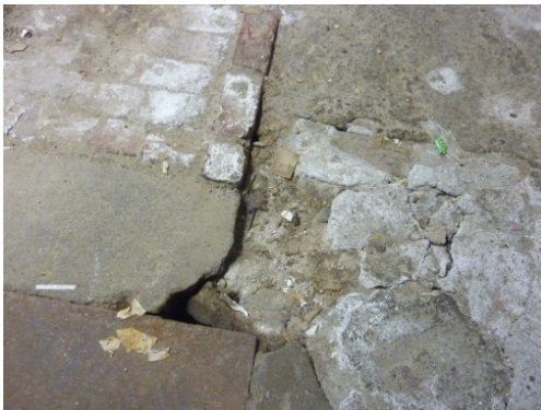
Original concrete, brick, and stone floor in center storage area of basement.
