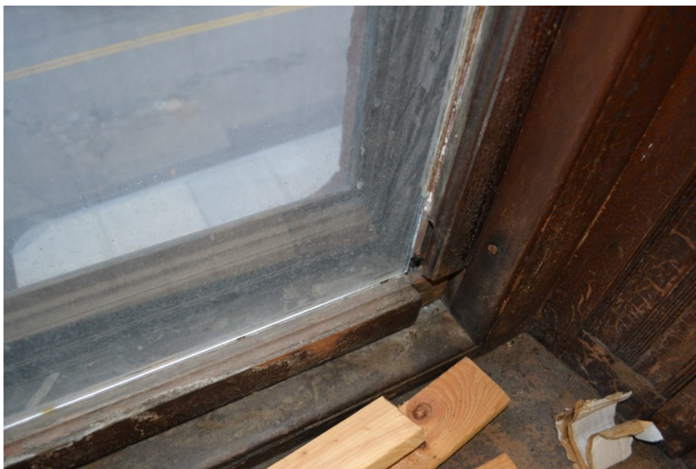
Broken wood sash at auditorium window.
