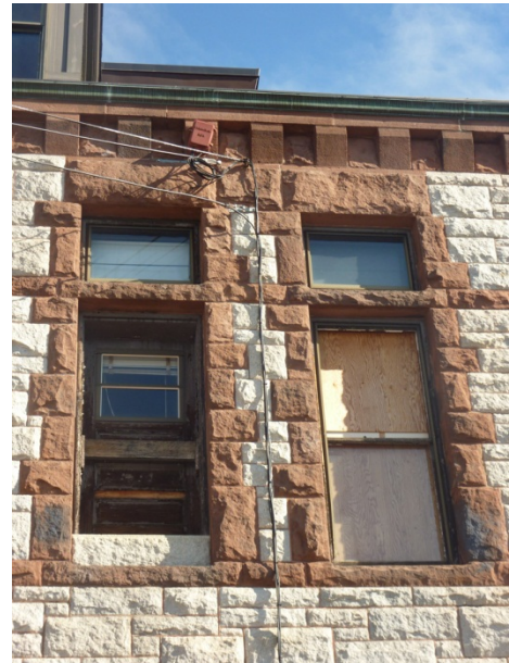
A range of window conditions exist.
