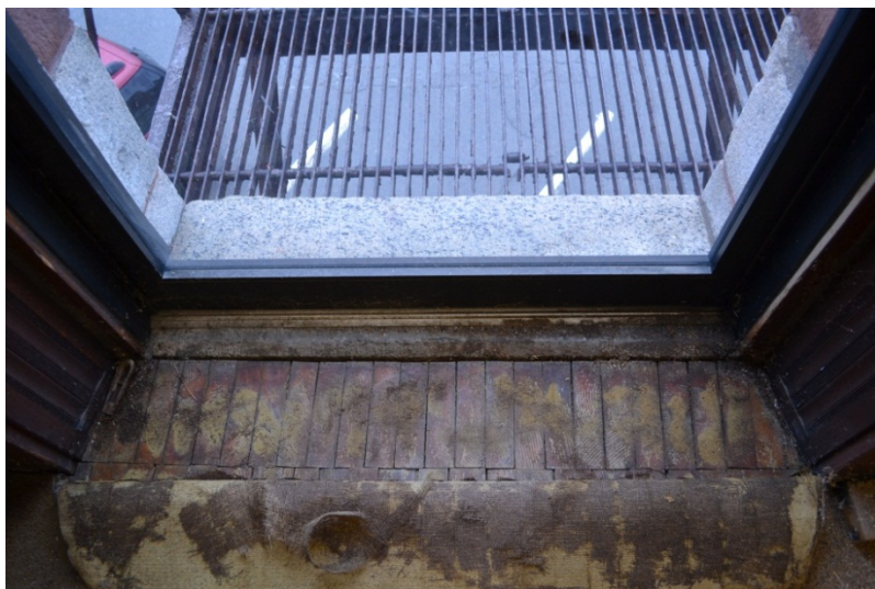
Emergency egress door at auditorium was a later addition
