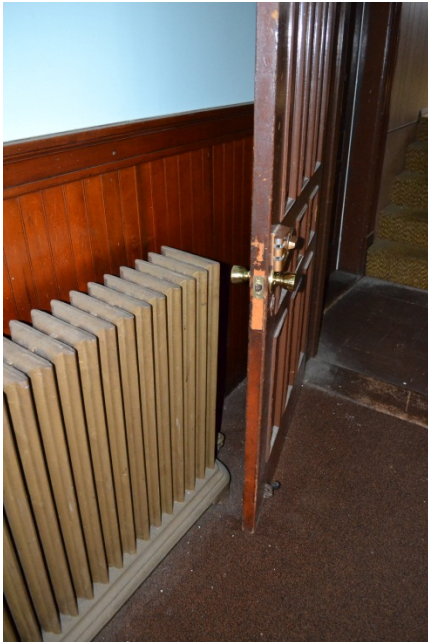
Door to backstage hits existing radiator when open
