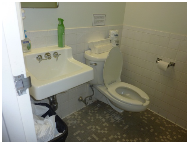
First floor inaccessible toilet room
