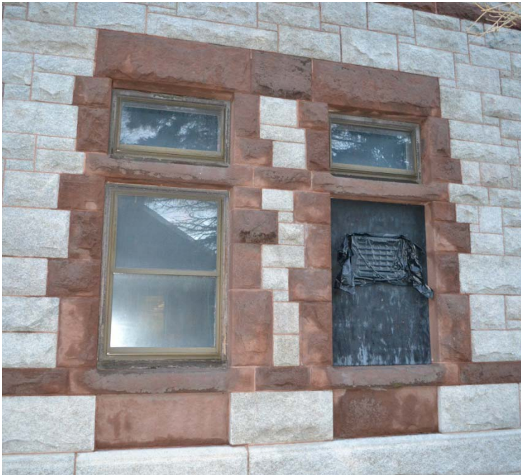
First floor east windows boarded from interior with wood veneer and exterior with plywood.
