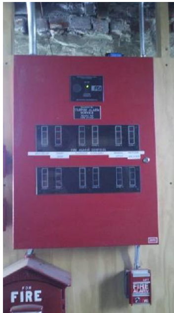
Figure 8 - Fire Alarm Panel
