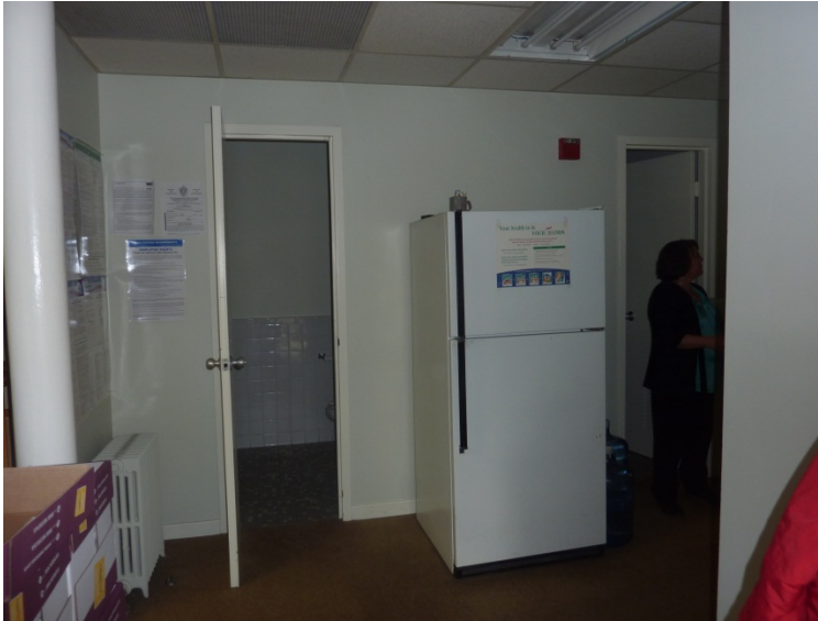
Doors to bathrooms do not meet minimum MAAB clearances
