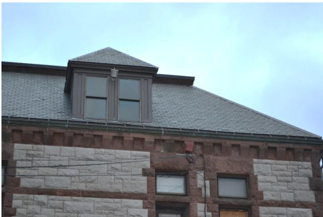
Worn gutters and missing slate on roof at south elevation.
