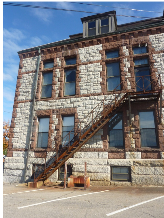
Rusting fire escape at south elevation.
