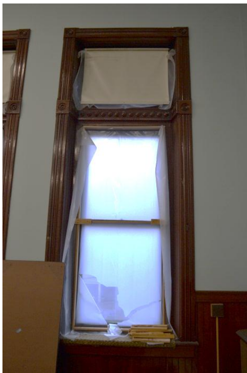
Interior of window at auditorium. Windows have temporary frames and plastic around them to keep out air infiltration.
