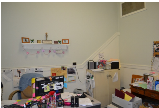
Location of original stairway from the stage elevation to the second floor
