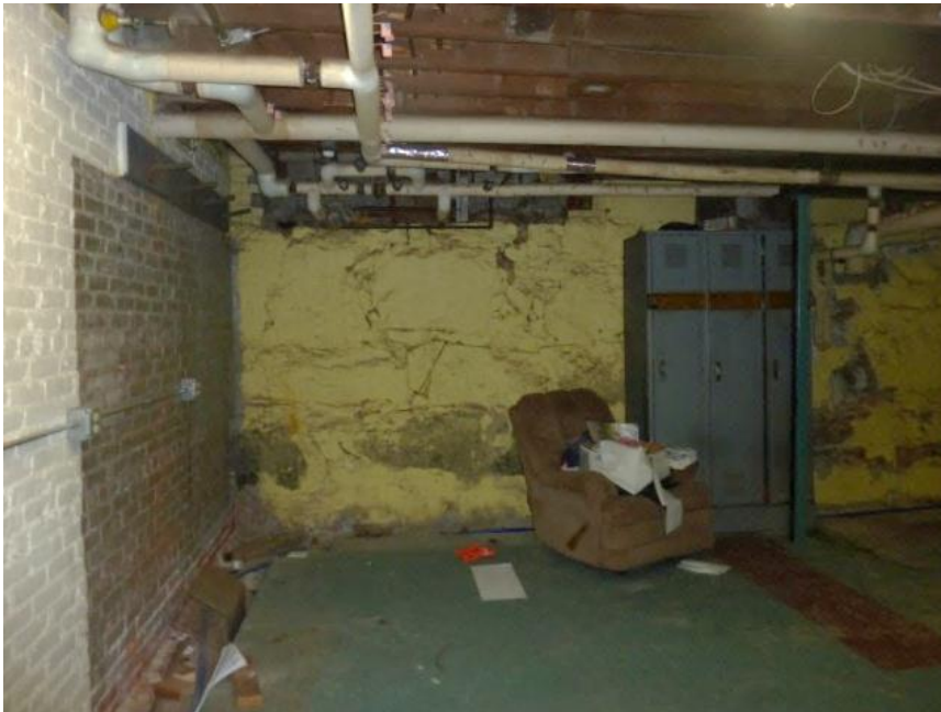
Stone exterior wall, brick load-bearing interior wall, and concrete floor in northeast storage room.
