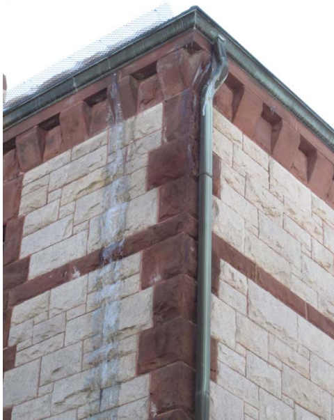
Frozen water at stone resulting from gutter leak.
