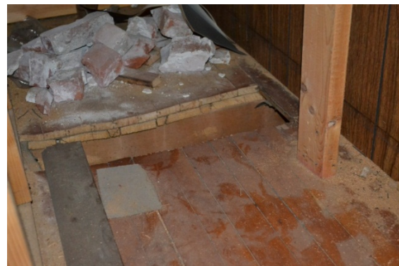
Under the stairs to the stage where the original wood floor and subfloor is exposed.
