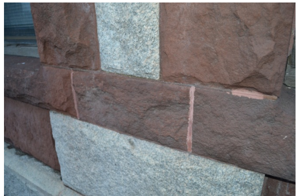
Incompatible mortar at a few stone locations.
