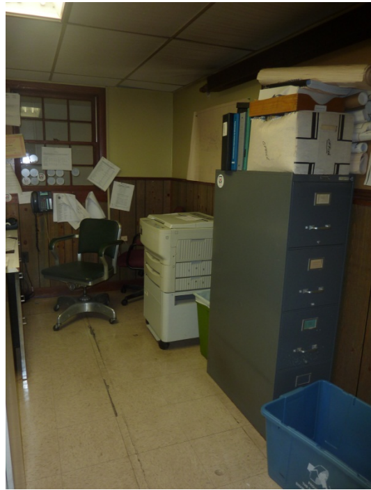
Vinyl tile chipping in Building Department office.
