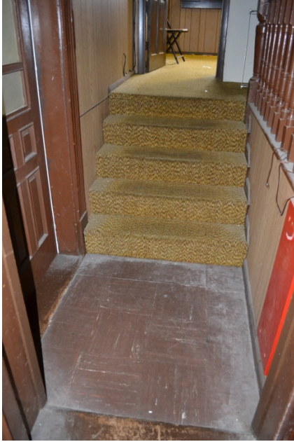
Stair to backstage does not have handrails
