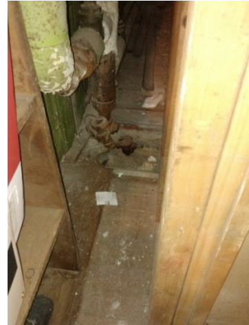
Steam pipe and grate at floor behind north wall in Board of Health office.
