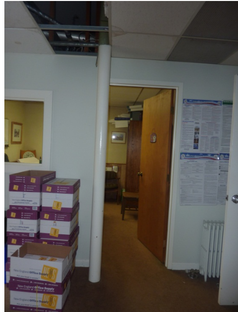
Original cast iron column blocks required clearances to Town Administrator's office.
