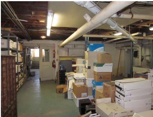
Pipe insulation at basement
