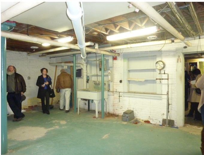
Painted concrete in northeast storage area.
