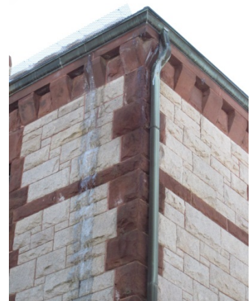
Water pouring under gutter at north elevation.
