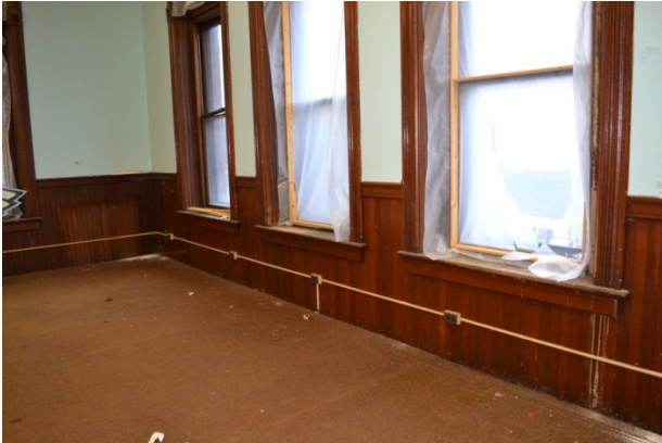
Electrical conduit at auditorium beadboard at exterior wall.
