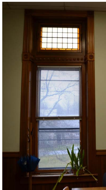
Interior of window at second floor conference room. Wood double hung sash and leaded glass in fair condition.
