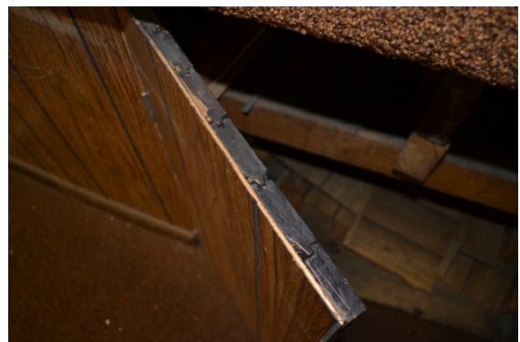
Tongue-and-groove beadboard wraps around stage walls, but has a layer of wood veneer applied to it.
