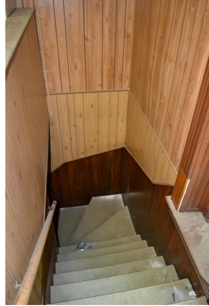
Southeast stair from first to second floor has winders and collides with the existing window.
