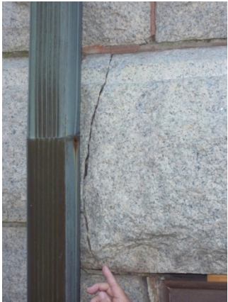
Large crack in granite above storefront window in basement
