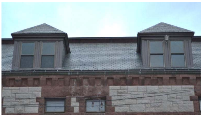
Staining on granite, worn gutters, and some missing slate at south elevation.
