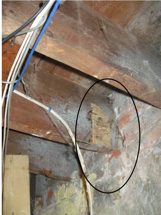
Figure 2: First Floor Joist End Deterioration at Exterior Wall
