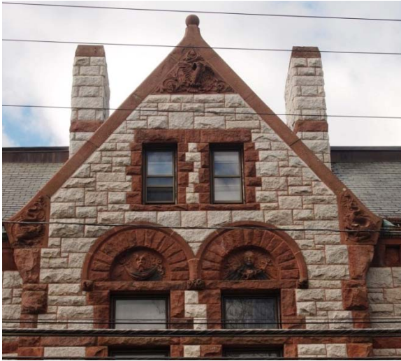
North elevation of granite carvings above windows, and at top and bottom of dormer.
