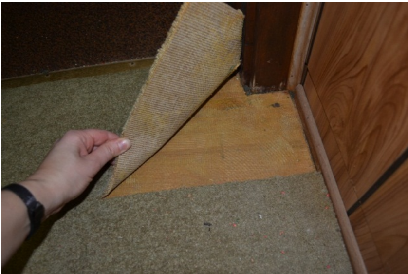
Plywood at floor under carpet at south storage room at stage level
