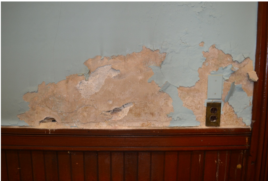
Deteriorating plaster on lath at west auditorium wall.
