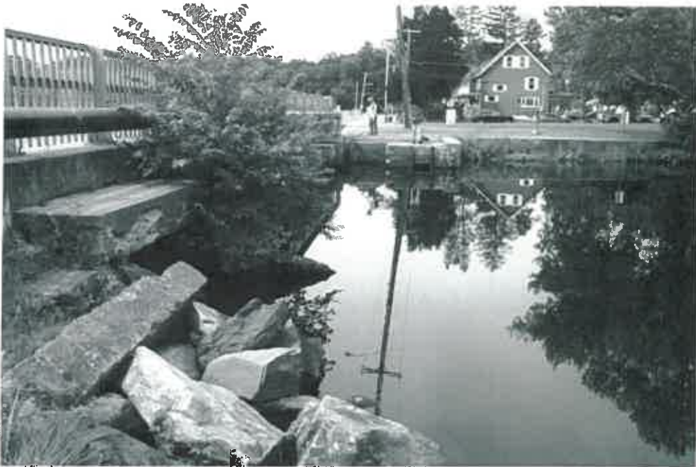
Photo 10 - Overview of bridge and dam from upstream; left outlet is in foreground
