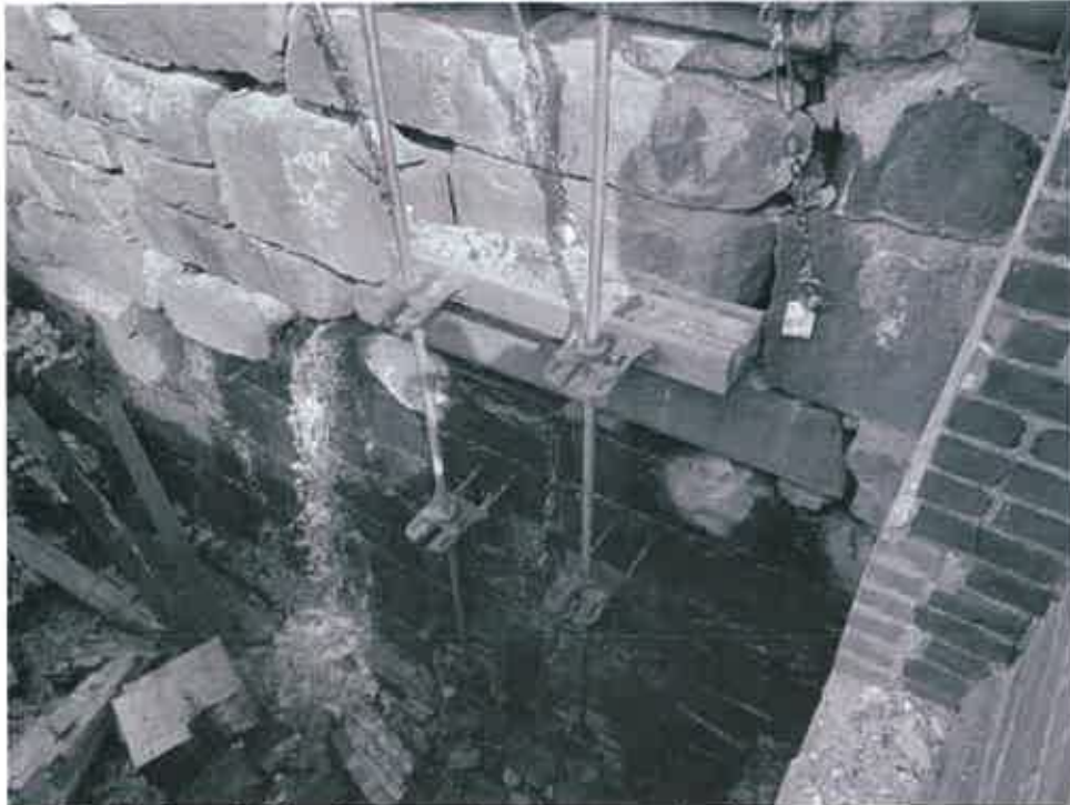
Photo 5 – Left outlet gate operator stems; note leakage through wall and missing mortar throughout wall
