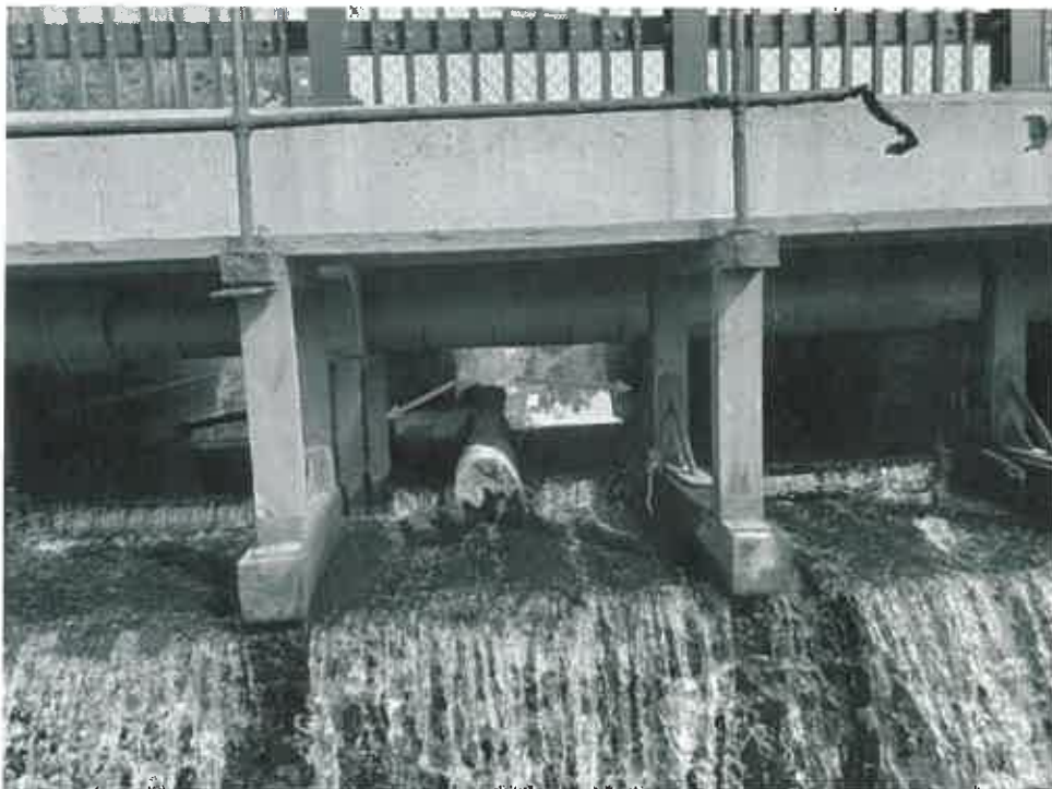
Photo 4 – View through Freedom Street bridge opening from downstream; note insulated water main; existing stoplog supports indicated with arrow; note debris within opening
