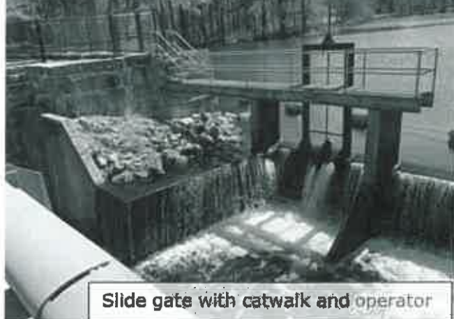
Leaning and deteriorated flashboards
