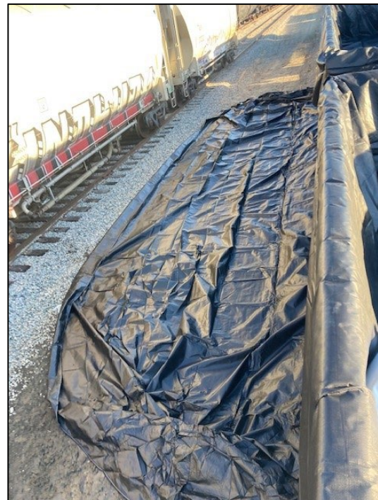
Figure 2. Photo of plastic sheeting used as intermediate barrier at the G&U Railyard
